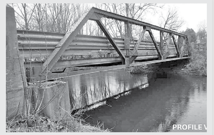
This historic bridge on Windham Concession 3 might replace the Porter Bridge at a cost of $500,000 to $600,000.
