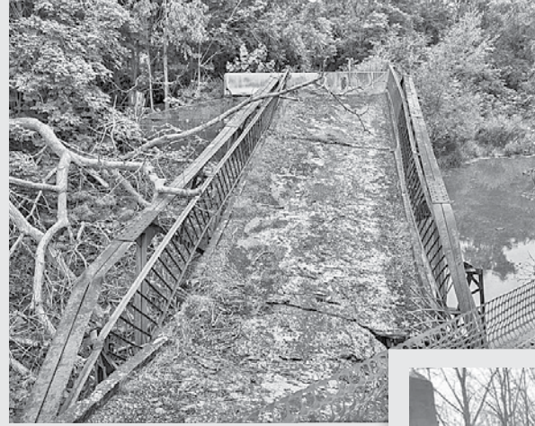
The Porter Bridge after it collapsed in August under its own weight.
